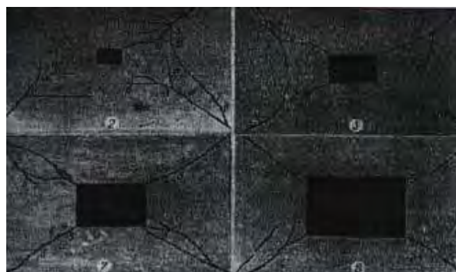
Fig. (8). A nature of development of cracks on four models of the elliptic paraboloid shells with different openings.
