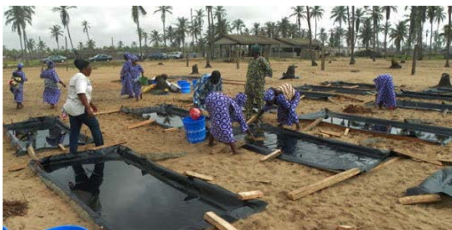
Figure 2. Photograph of women Association of Sèmè-Okoun installing the salt production plant which's fundamental component is the black tarpaulin held by woodbin.
