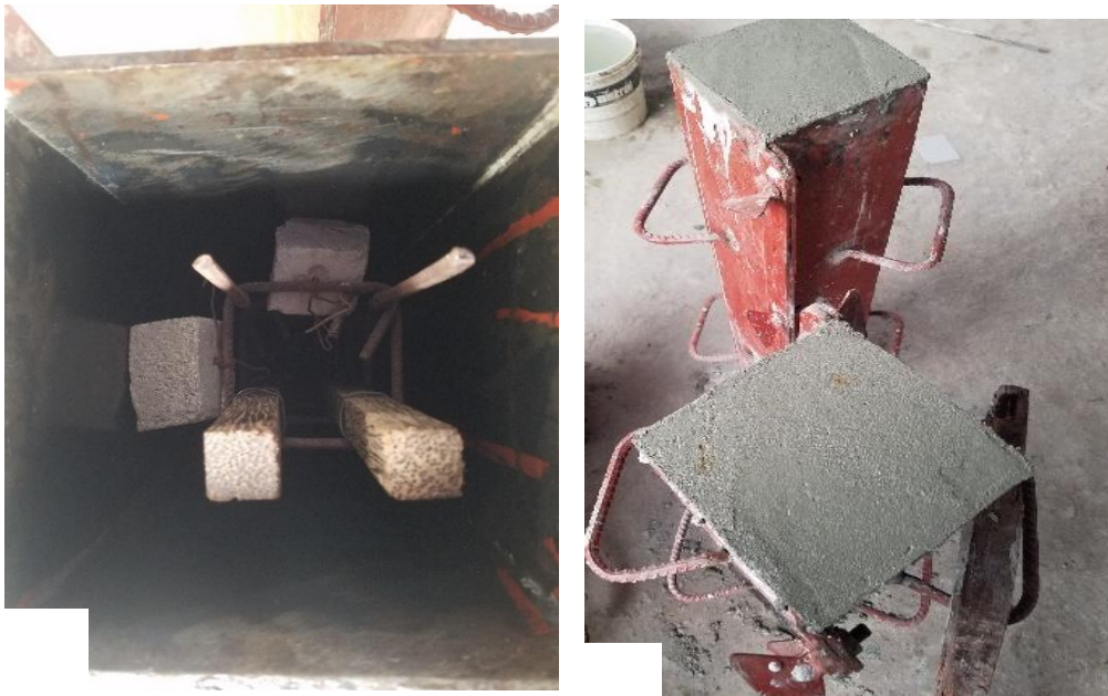
Figure 03:- Appearance of the beams during casting: a) Reinforcement of the beam in the mould b) Appearance of the beams cast in the mould.
