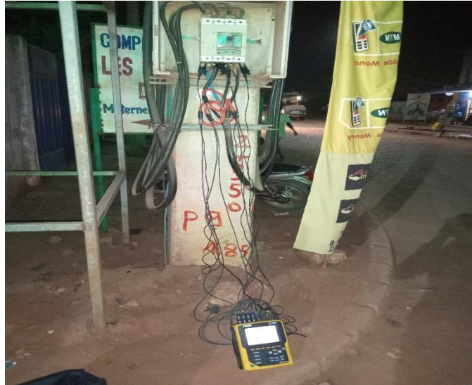
Figure 2: View of analyzer installation for measurements.
