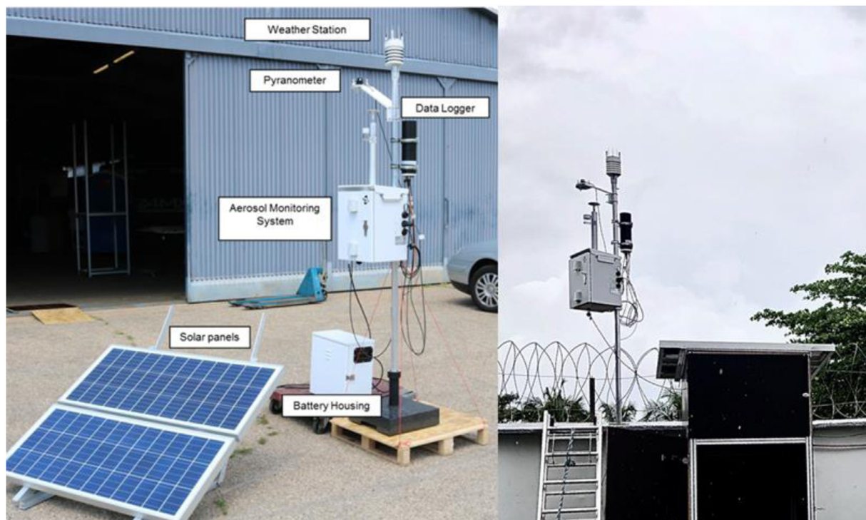
Fig. 1. Left - photograph of the assembled monitoring equipment before it has been shipped from Karlsruhe (Germany) to Cotonou (Benin). Right - Photograph of the monitoring equipment positioned at the top of a Pylon over the Boulevard de la Marina in Cotonou)
