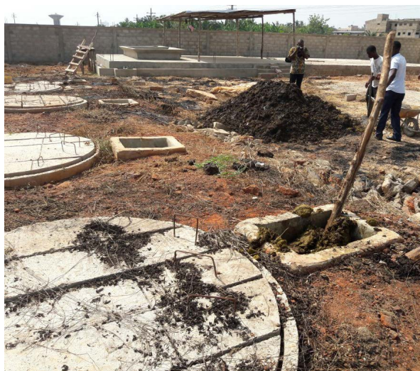
Figure 5. Methanization and biogas production disposal in Lomé (Photos: E. Chokpon, July 2020).
